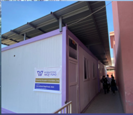
Four toilet blocks were repaired and upgraded – two for teachers, and two for students
